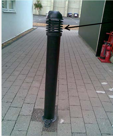
Air temperature bollard installed above the GSHP tank
